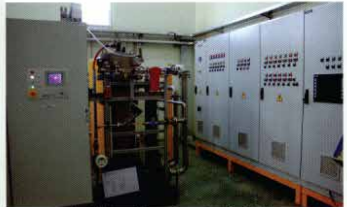
Installation of Ozone Generators (2 x 2 kg/h)
